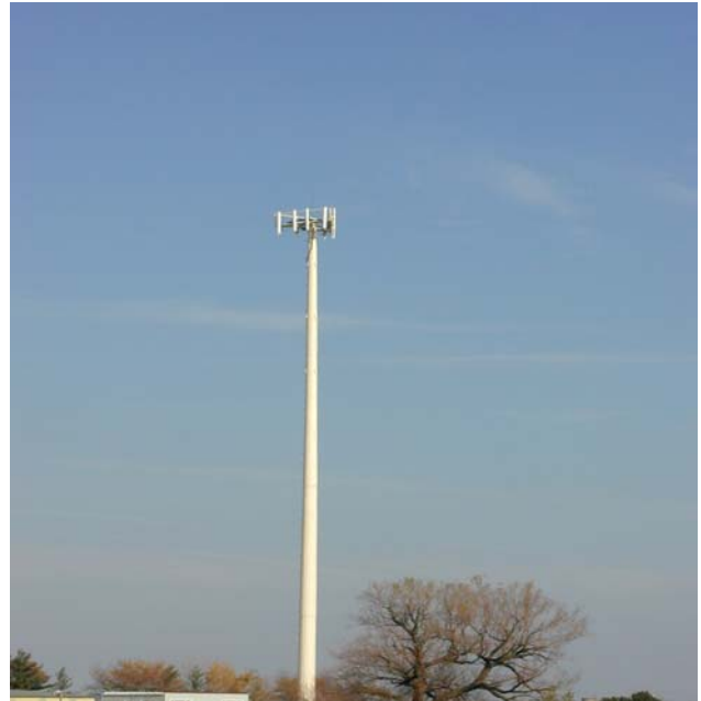
Single-carrier poles were the first built and, therefore, typically have premier locations.
